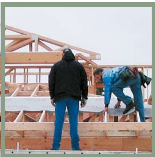
SolAire Homebuilders and DuPont employees install the AtticWrap on Vidas' home. Photo by Cindi O'Neil.
